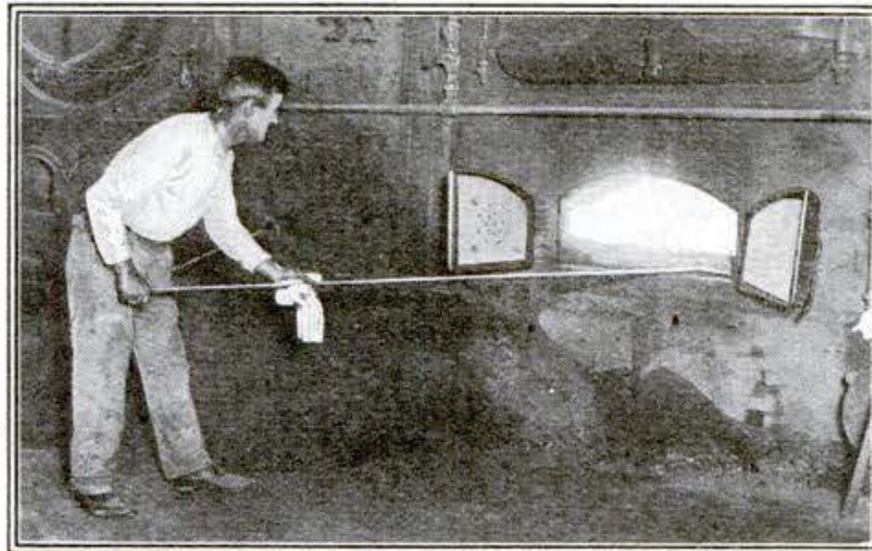
The composition fuel in use. The ash on the floor in front of the boiler shows freedom from clinker and a free-burned granular condition
